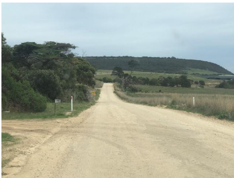
North Coast Road 4 - typical condition
