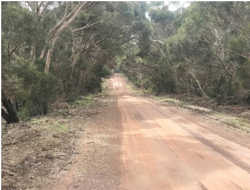
Rose Cottage Road 1 – typical condition
