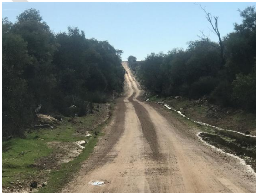
McBrides Road 2 - insufficient drainage
