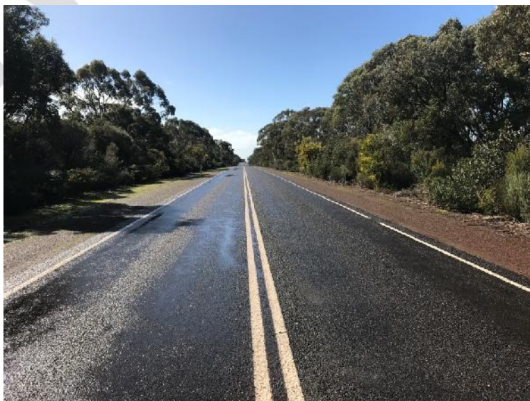
Playford Highway 4 - evidence of seal delaminating
