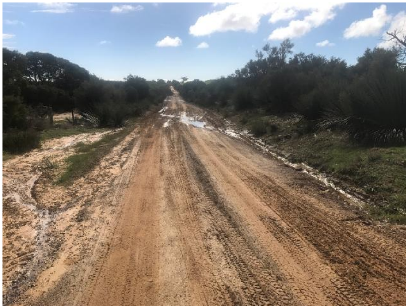
McBrides Road 1 - typical condition (poor)
